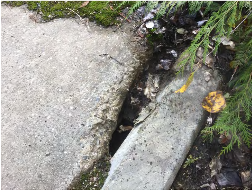
Damage to panel 1 at left approach
