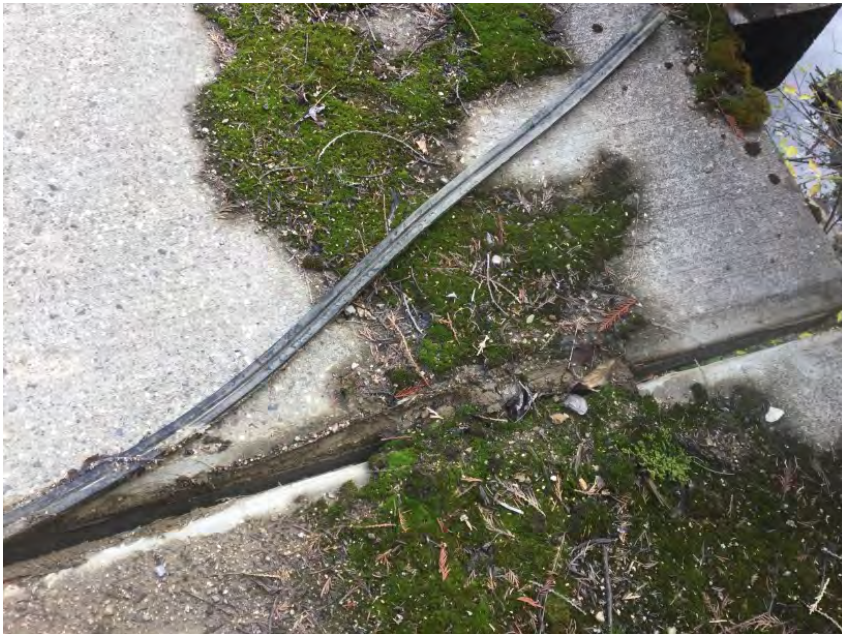
Deck seals not functional
